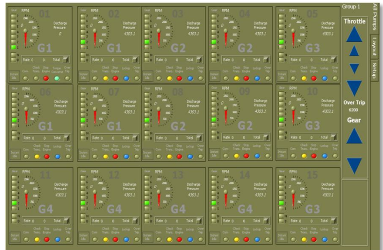
Multi-Pump Control Screen
